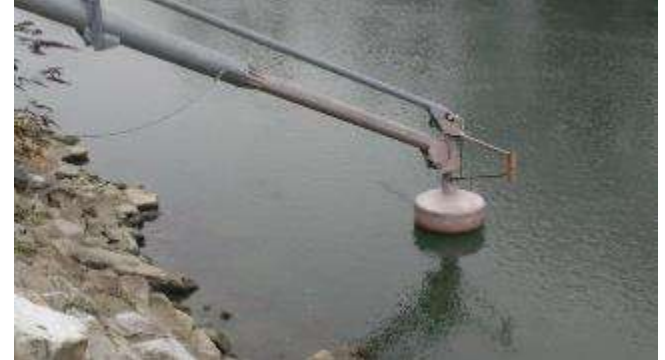
Veolia , drinking water facility, River Pumping station
