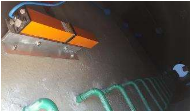
Water Plant , St Etienne
