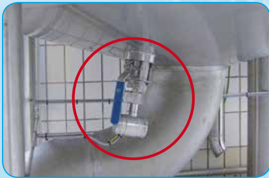
2000-VALVE, Code W110 in tank bottom
